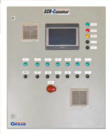
Control and Logger Unit
