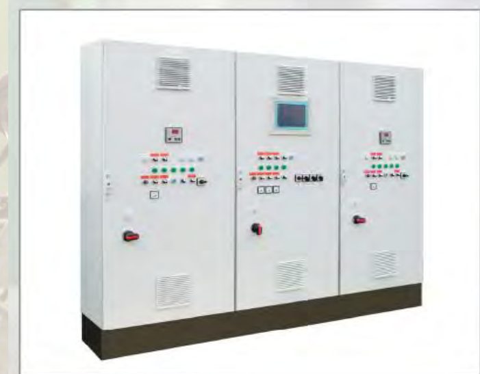
Fig: Typical Control Cabinet
