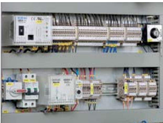
BMS safety devices.
