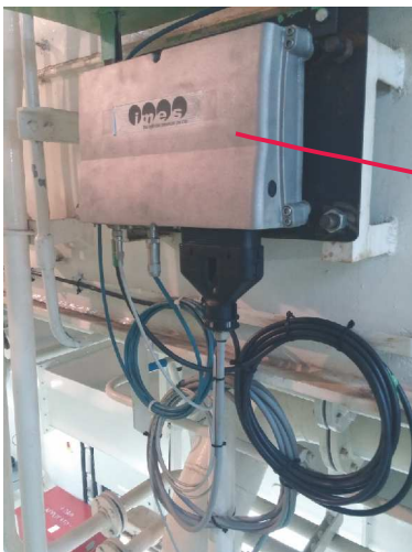
CCM Marine performance installed on container ship Hedda Schulte
